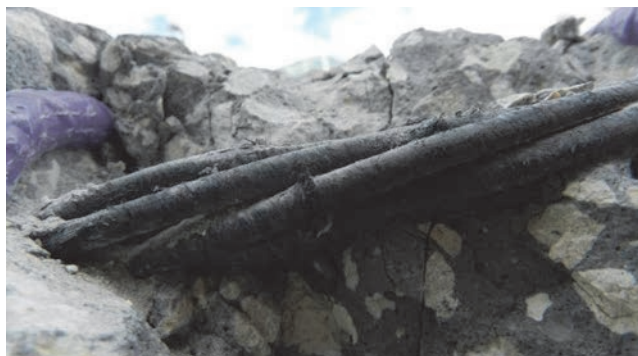
Figure 17. Rupture of the strand after chipping
