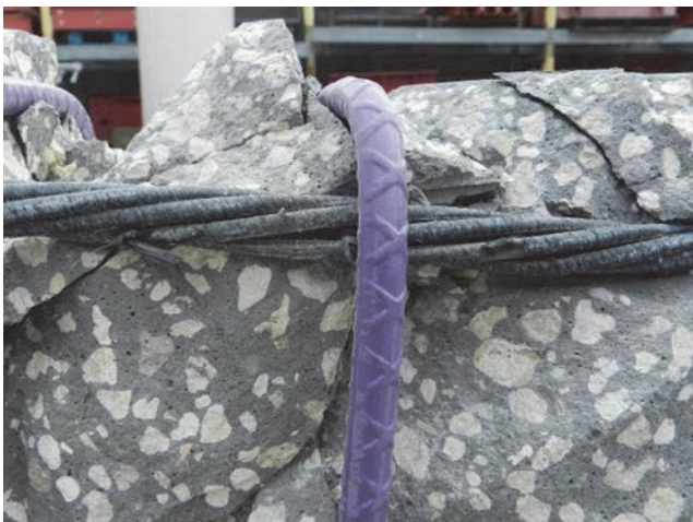
Figure 22. Specimen after chipping
