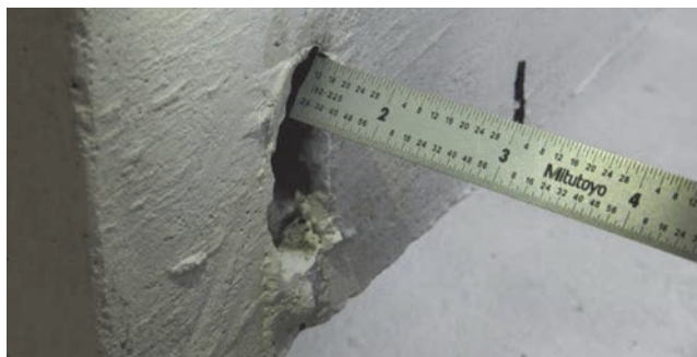
Figure 16. Slippage at right end of front CFCC strand
